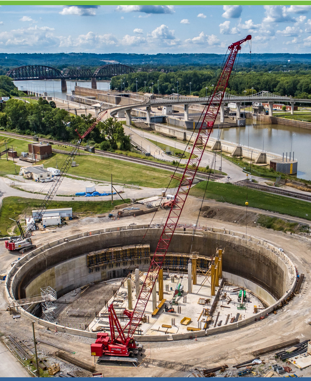
Construction continues on the Portland Combined Sewer Overflow Basin located in Lannan Memorial Park.
